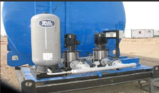
Hydropneumatic Pressure Booster Pumps
