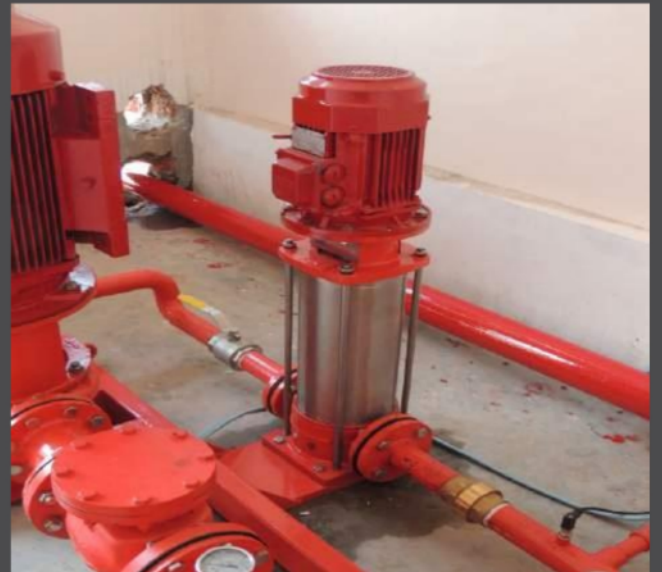
Jockey Pump fitted in Fire Fighting System.
