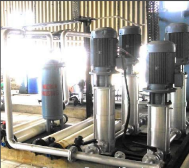
High Pressure Pumps.(Combo) Pressure: 60 Bar. Flow: 90 M 3 /Hr
