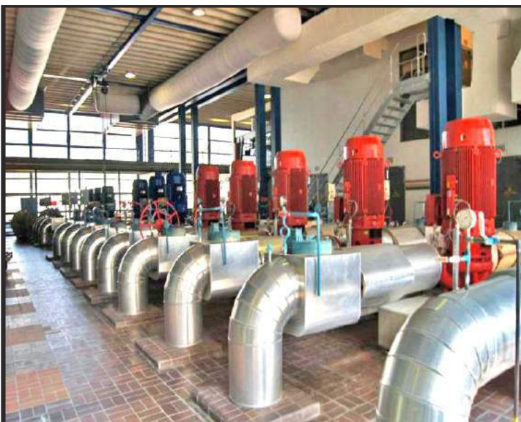
IN-LINE PUMPS WORKING AT A.C PLANTS
